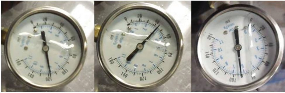
FIG. 2: MEASUREMENTS AT NO FLOW, FULL FLOW RESTRICTED, AND FULL FLOW OPTIMIZED
